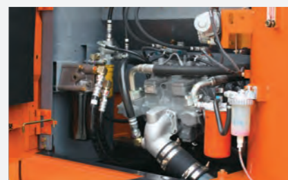
Grouped remote filters and inspection points
